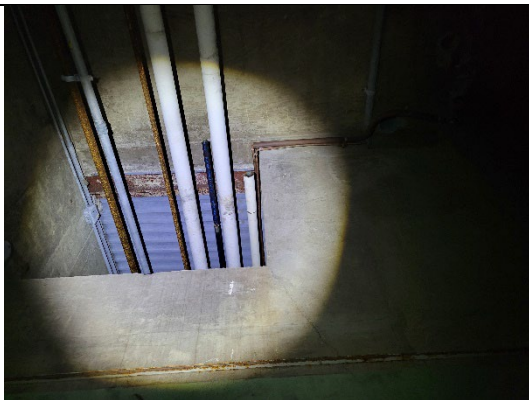
Pipes, wrapped and painted, running through the roof of the first floor. Room to the east of the elevator mechanic room.
