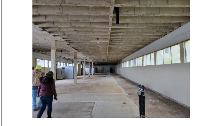
Main room on the first floor, facing east toward the entrance to the generator and elevator rooms.
