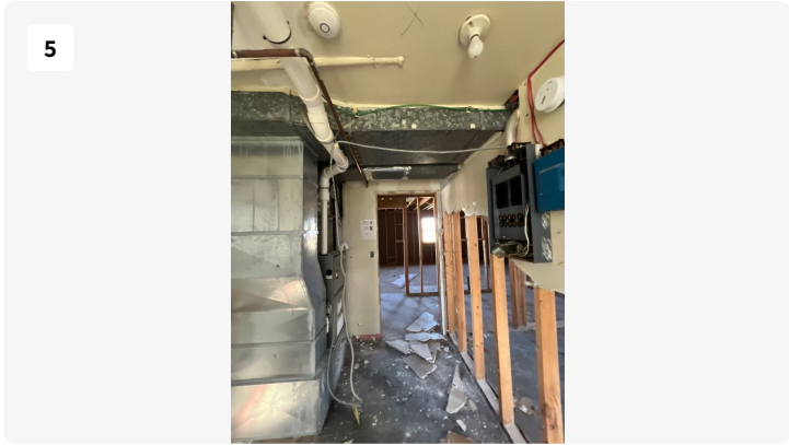
Project: Blackstone-house Date: 3/11/2024, 9:32am Creator: Logan Drake Tags: Basement utility
