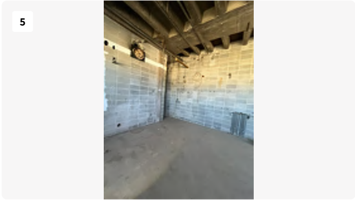
Project: Blackstone-hospital Date: 3/11/2024, 11:45am Creator: Logan Drake Tags: Rm 120 Electrical
