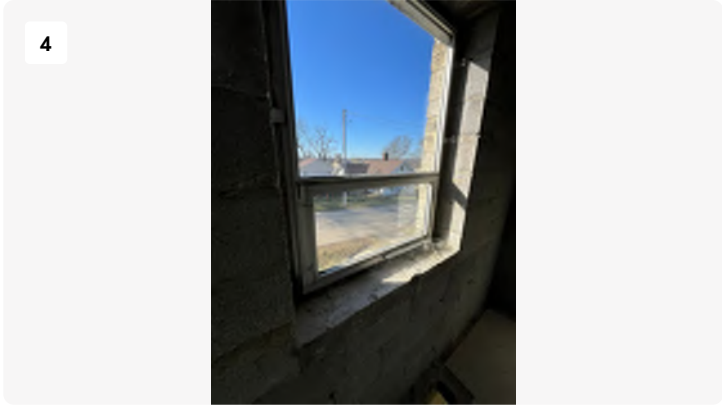
Project: Blackstone-hospital Date: 3/11/2024, 10:04am Creator: Logan Drake Tags: 2nd floor North open
