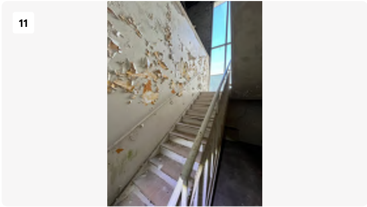
Project: Blackstone-hospital Date: 3/11/2024, 12:06pm Creator: Logan Drake Tags: SW stairwell to 2nd
