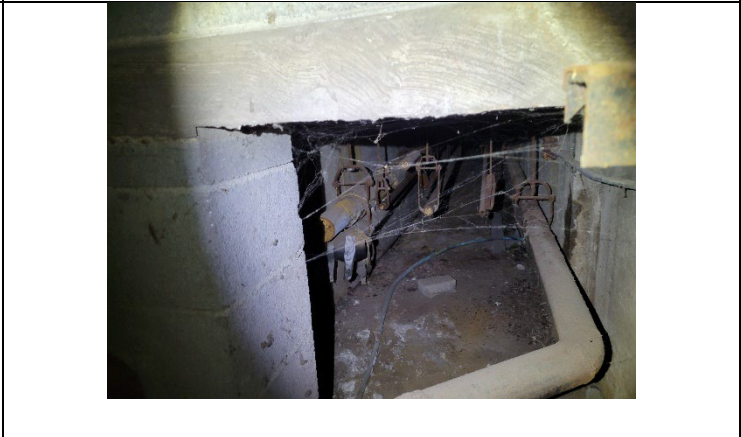
Crawl space entrance within the diesel generator room. Entrance is within generator room in the northwest corner.
