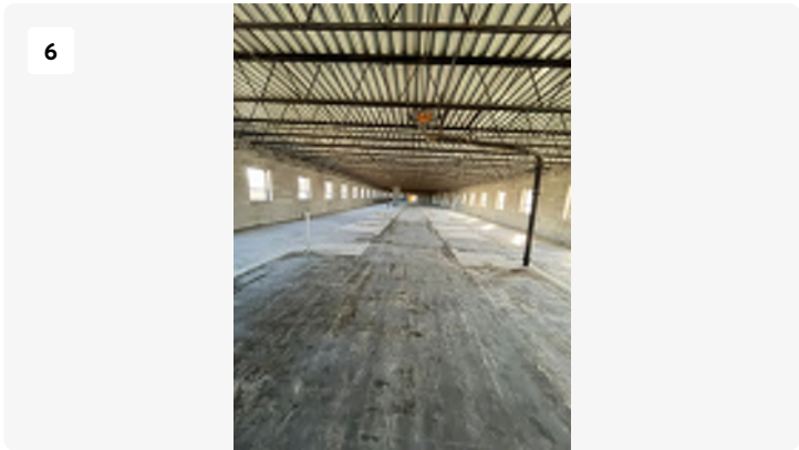
Project: Blackstone-hospital Date: 3/11/2024, 10:04am Creator: Logan Drake Tags: 2nd floor North open
