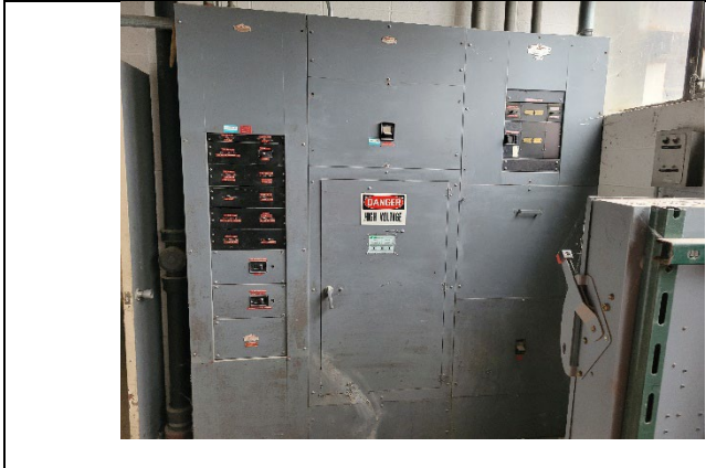
Electrical panel in the old diesel generator room located in the northeast corner of the first floor.
