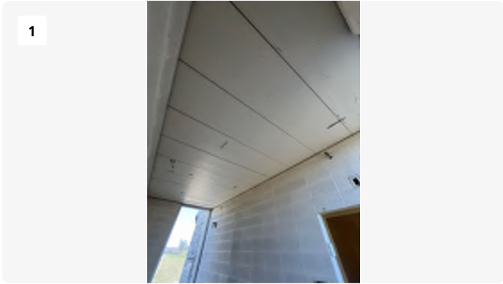
Project: Blackstone-hospital Date: 3/11/2024, 10:01am Creator: Logan Drake Tags: west stairwell to 2nd
