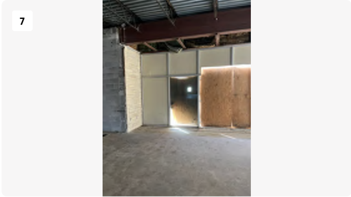
Project: Blackstone-hospital Date: 3/11/2024, 10:38am Creator: Logan Drake Tags: 2nd floor South Open
