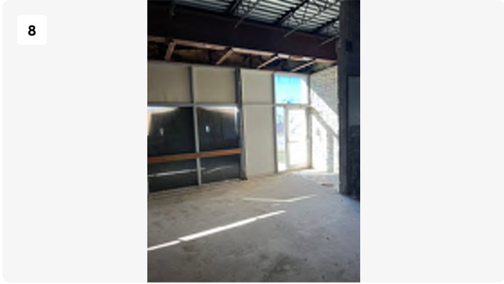
Project: Blackstone-hospital Date: 3/11/2024, 10:38am Creator: Logan Drake Tags: 2nd floor South Open
