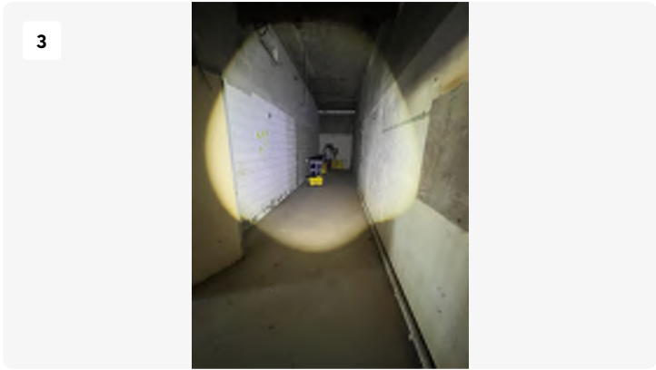
Project: Blackstone-hospital Date: 3/11/2024, 10:57am Creator: Logan Drake Tags: 1st floor Storage A
