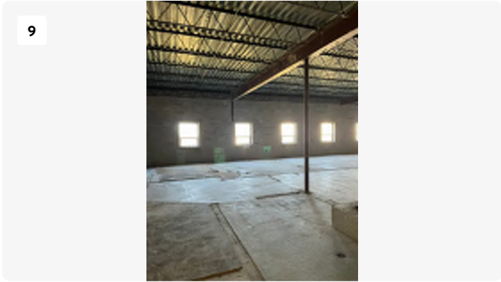
Project: Blackstone-hospital Date: 3/11/2024, 10:38am Creator: Logan Drake Tags: 2nd floor South Open
