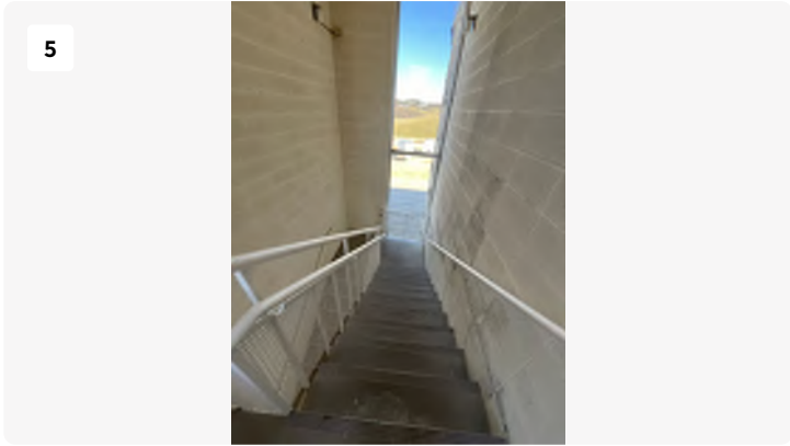
Project: Blackstone-hospital Date: 3/11/2024, 10:01am Creator: Logan Drake Tags: west stairwell to 2nd
