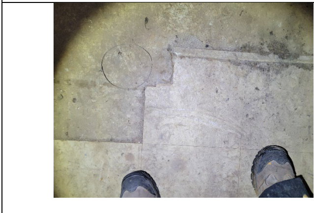
Vinyl floor tile on top of sheet flooring on the first floor.
