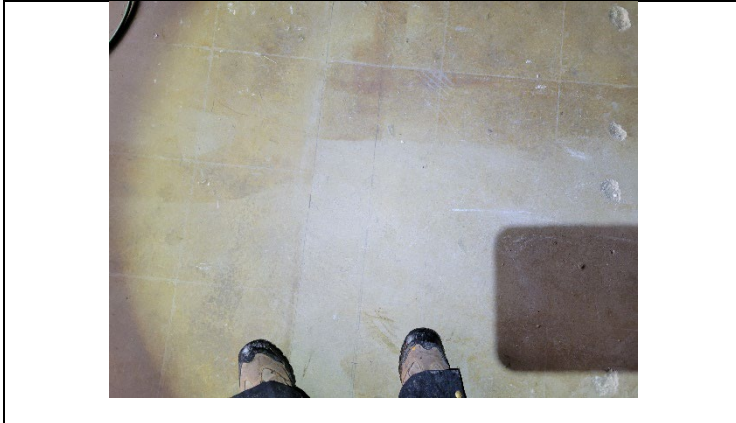
Residual glue on floorboards on the second floor of the residential structure.
