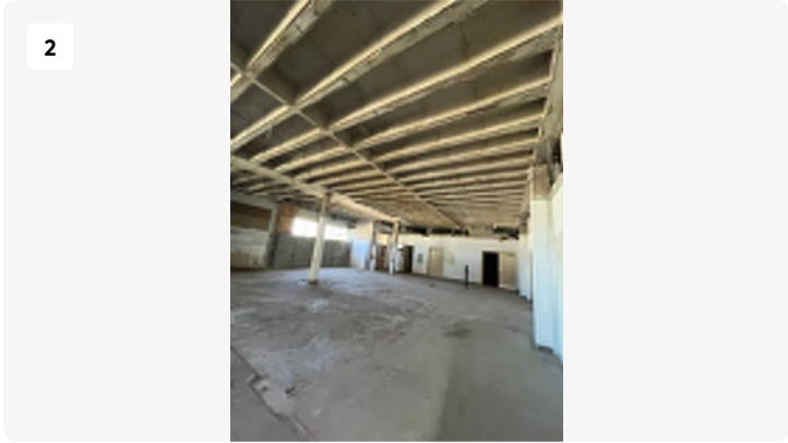
Project: Blackstone-hospital Date: 3/11/2024, 12:06pm Creator: Logan Drake Tags: 1st floor open space
