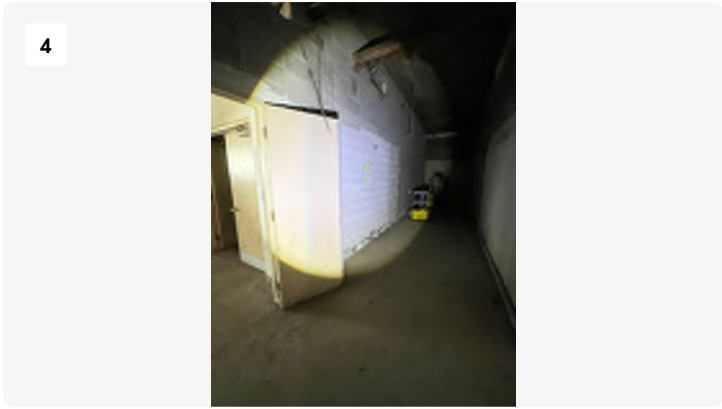
Project: Blackstone-hospital Date: 3/11/2024, 10:57am Creator: Logan Drake Tags: 1st floor Storage A
