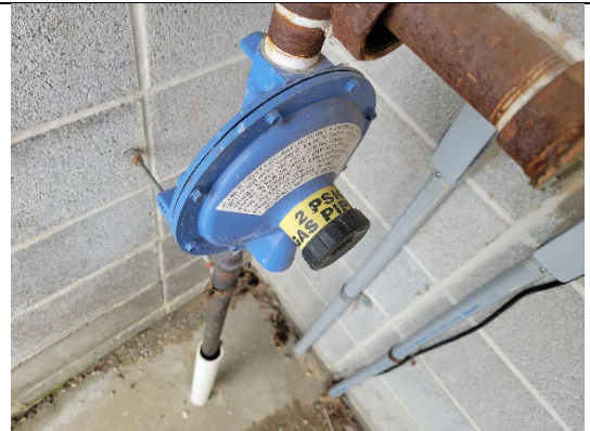
Gas service line within the gated alcove.
