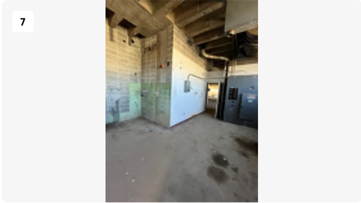
Project: Blackstone-hospital Date: 3/11/2024, 11:45am Creator: Logan Drake Tags: Rm 120 Electrical
