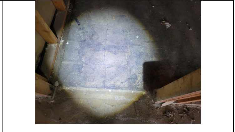
Tiles on the first floor in the room with the water heater. Room to the east of the stairs down.
