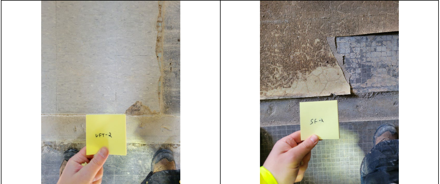
Vinyl Floor Tile – 2, Picture taken east of the stairwell on the second floor black mastic – 5% chrysotile. Note, this mastic was observed throughout the second floor without tile. Sheeting Floor – 2, picture taken west of the south entrance to the second floor – black backing/mastic – 65% chrysotile.
