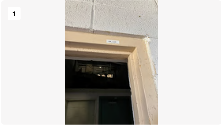
Project: Blackstone-hospital Date: 3/11/2024, 11:45am Creator: Logan Drake Tags: Rm 128 Mens Restroom 1st floor
