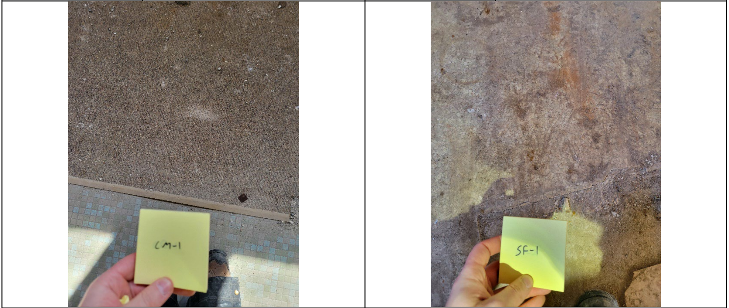
Carpet Mastic – 1, picture taken on the south wall of the first floor – yellow and black mastic: black mastic – 5% chrysotile, yellow mastic - <1% chrysotile. Sheet Flooring – 1, picture taken west of the north entrance to the first floor – black backing/mastic – 65% chrysotile.
