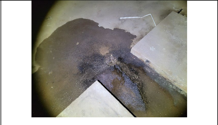
Floor drain in the diesel generator room with stained concrete.
