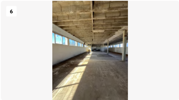
Project: Blackstone-hospital Date: 3/11/2024, 12:06pm Creator: Logan Drake Tags: 1st floor open space
